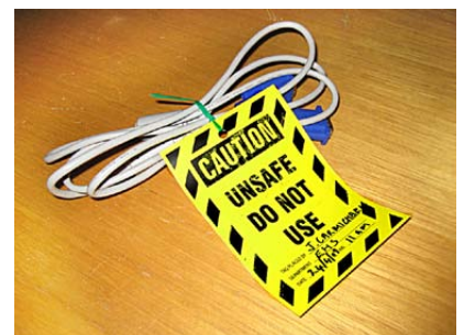
Damaged cable tagged out
