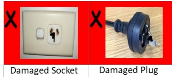
Damaged electrical socket-outlet and plug
